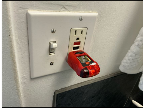
GFCI in place and operational.
