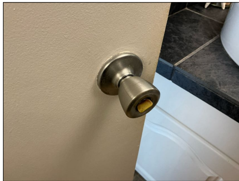
Doorknob does not lock properly. Recommend replacing.
